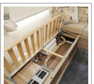
THE SEAT OF POWER The offside seat box has to accommodate the battery box and the electrical MCU, seen on the left, which is accessible and easy to use
