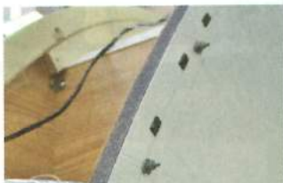
A new feature involves drilling into the sidewall in order to fit these plastic fir-tree fixings upon which the awning rails are now bonded. This is a new process
